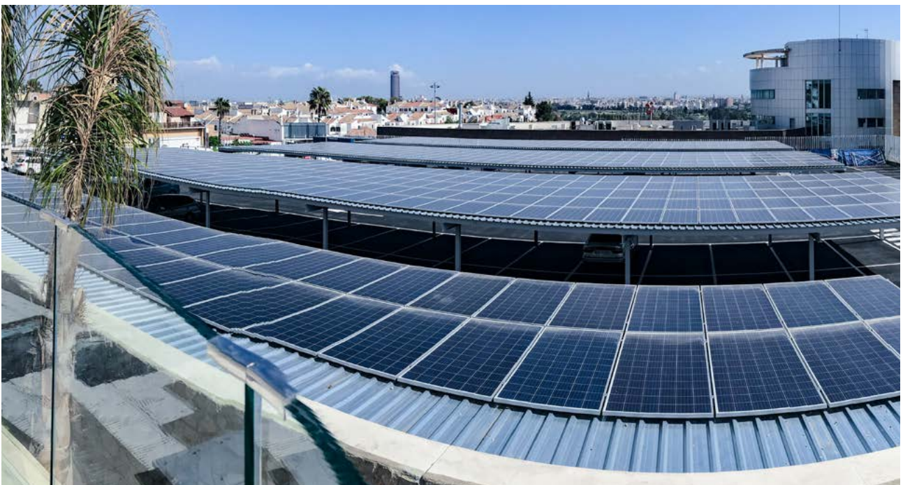
Solar panel system at the Gran Casino Aljarafe in Seville
